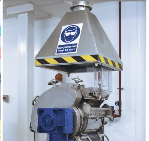
FT32-20 Vapour extraction system
