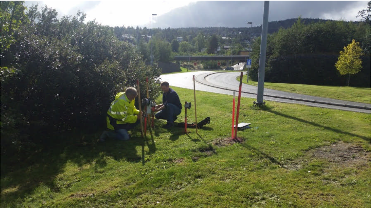
Fig. 7 – Remote read-out solution example: Monitoring of pore pressure in clay at different depths under a road. The gateway receives settings and sends logged data via the mobile phone network.
